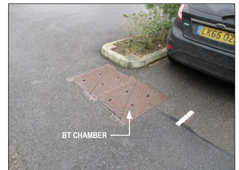
PHOTOGRAPH 3 EXISTING BT CHAMBER IN CAR PARK AREA ADJACENT TO BUILDING 1/2
