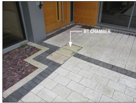
PHOTOGRAPH 5 EXISTING BT CHAMBER IN PAVED AREA OUTSIDE ENTRANCE TO BUILDING 5
