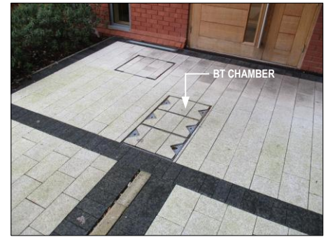
PHOTOGRAPH 6 EXISTING BT CHAMBER IN PAVED AREA OUTSIDE ENTRANCE TO BUILDING 4
