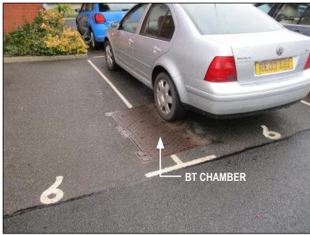
PHOTOGRAPH 4 EXISTING BT CHAMBER IN CAR PARK AREA ADJACENT TO BUILDING 5/6
