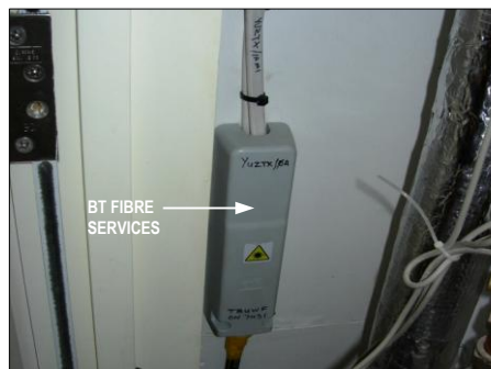
PHOTOGRAPH 8 BT FIBRE GAS SEAL IN GROUND FLOOR RISER IN BUILDING 4
