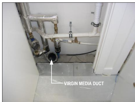
PHOTOGRAPH 11 VIRGIN MEDIA DUCT ENTRY TO GROUND FLOOR RISER IN BUILDING 6
